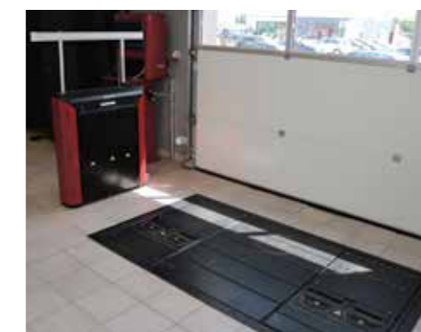
Bosch Car Service Viborg's tyre hotel has space for 1000 wheelsets and the workshop has tyre scanning equipment from HUNTER
