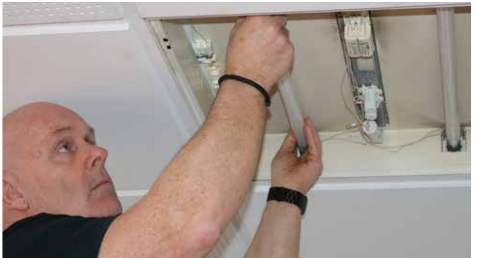
Jørn K. Jensen is switching to LED lighting, which has resulted in an annual saving of more than 40,000 kWh
